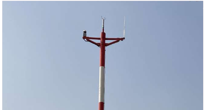
Ultrasonic Anemometer Mounted on a Frangible Mast
